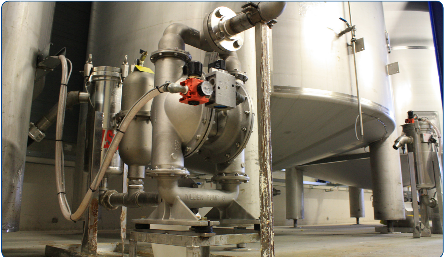
A stainless-steel Wilden® Advanced™ PX Series AODD Pump in use at the SABA B.V. glue- and adhesive-manufacturing facility in The Netherlands.
