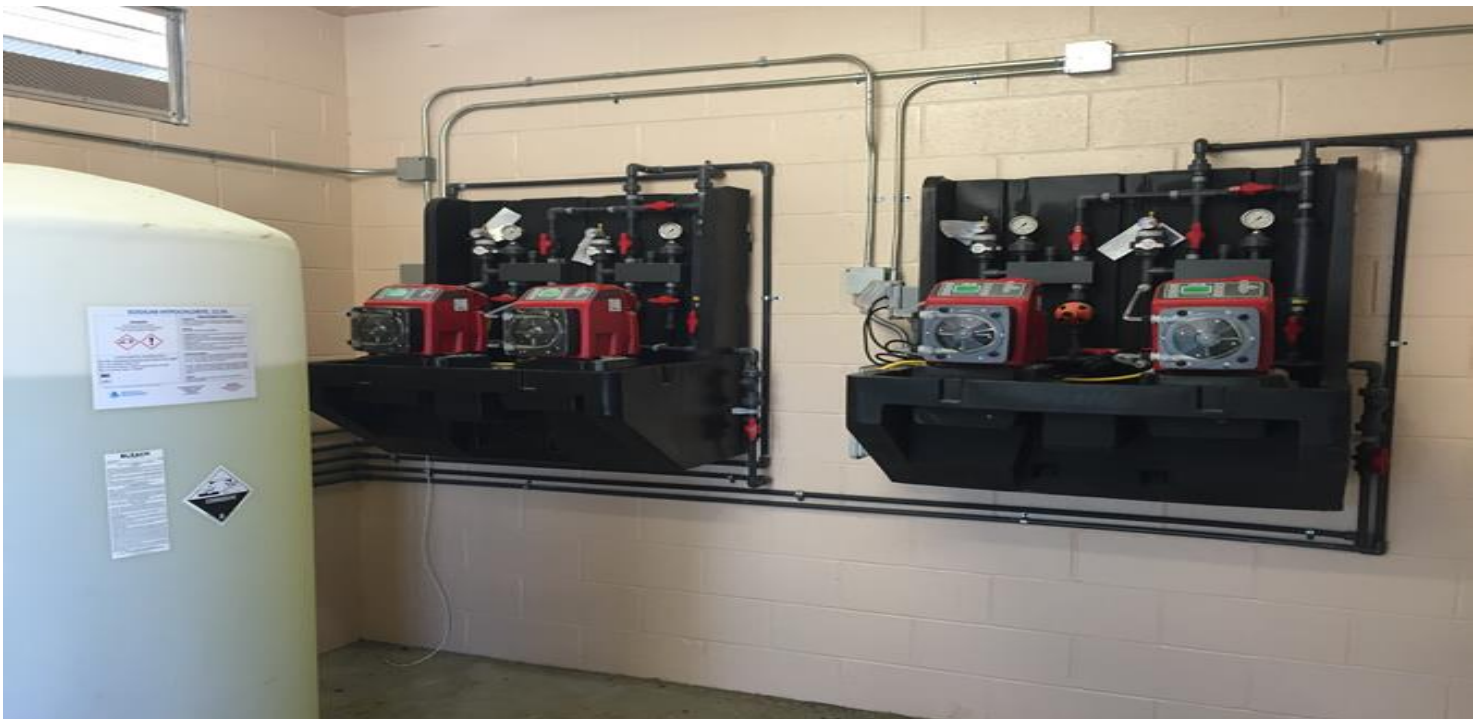
Fig. 2: Flowrox Packaged Pump Systems installed at Camden, TN waste water facility
