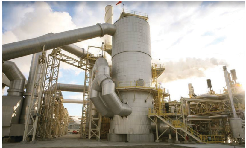
Evaporation system with subject pumps and seals.
