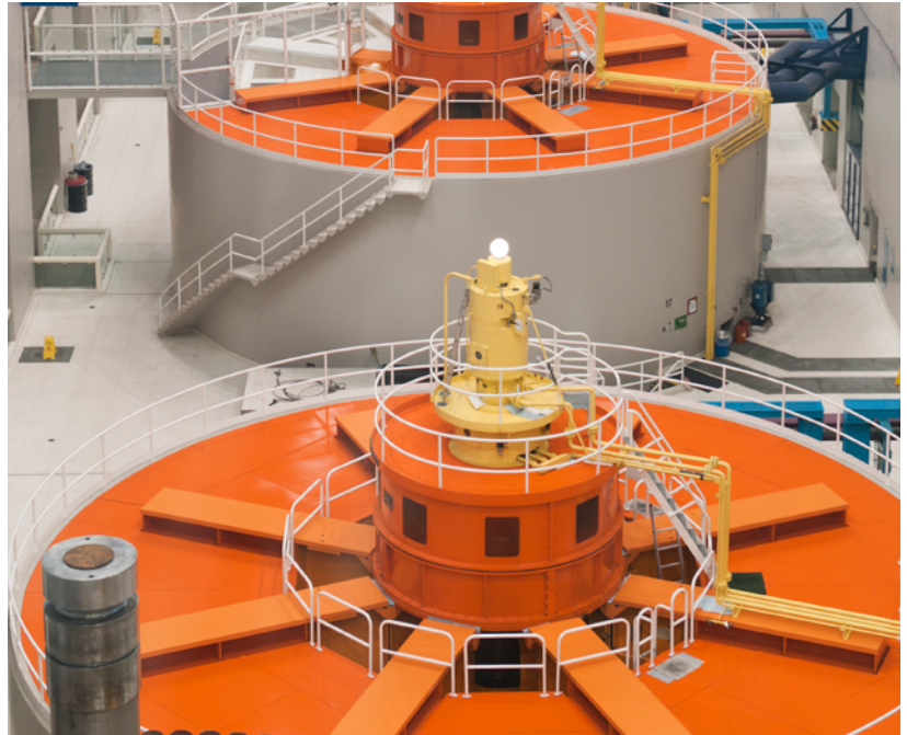
Maintaining high reliability of equipment requires monitoring performance and condition.
